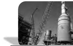
Plant Inspection & Testing
